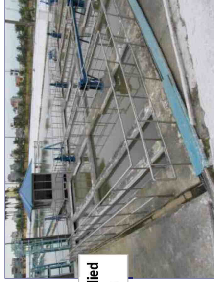
Main water treatment plant (An Duong Water Treatment Plant)
